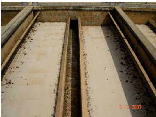
Figure 3. Comparison between the sand filter tank (before) and the retrofitted membrane tank (after)
